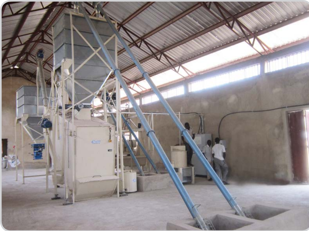
▲ Discharge augers from concrete sumps deliver pre-ground raw material to weighing hopper mounted above mixer.
