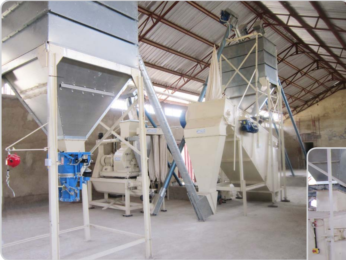
Sacking hopper with weigher, gravity discharge high performance hammermill and batch mixer with overhead weighing hopper ▲
