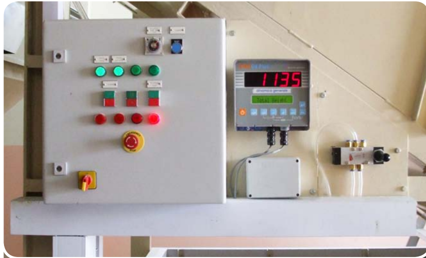
◀ Control panel and digital weight controller with large display
