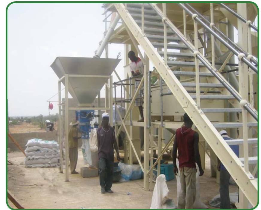
▶ Side view of the Plant during initial test run.
