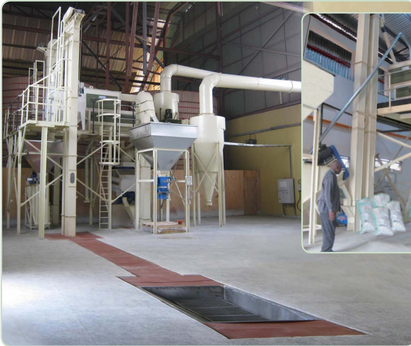
▲ The complete sorghum cleaning and destoning plant with grain reception conveyor in the foreground.
